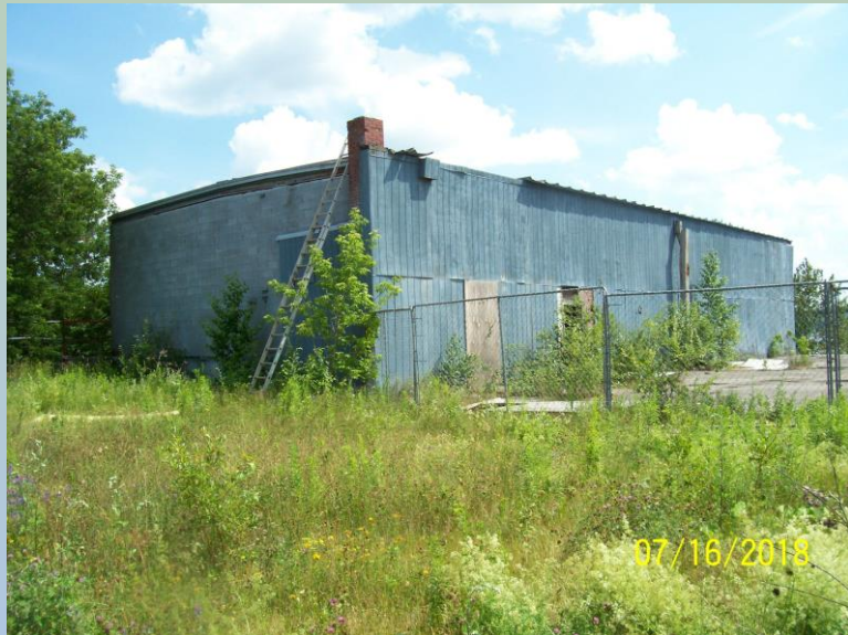
Blighted and Dangerous Industrial Building: Colby Starch Plant
