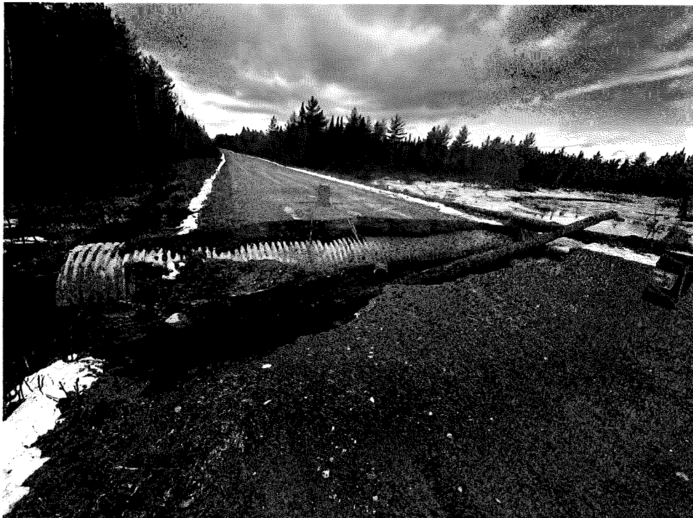
Stud Mill Road is impassable in TWP32 after the December 18 th storm. Numerous Bear Hunting Leases are accessed off Studmill Road.
