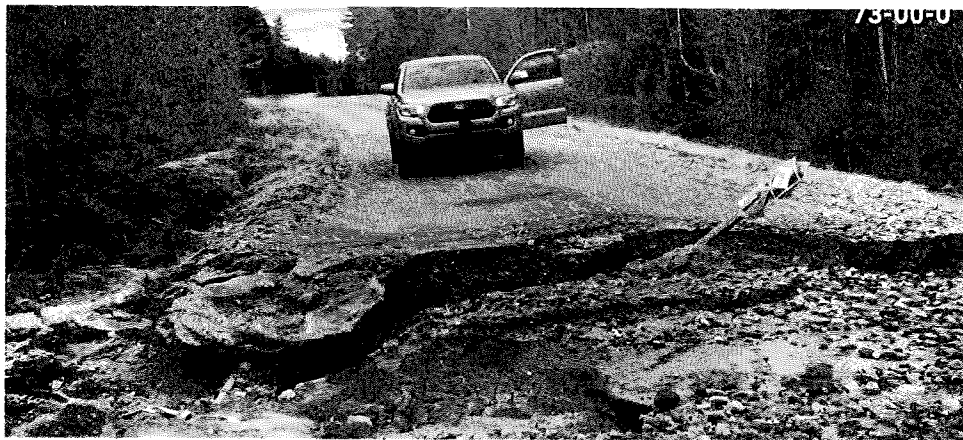
73-00-0 Road in Osborn TWP, road washed after December 18 th . Note the sign indicating the road is also an ATV trail.
