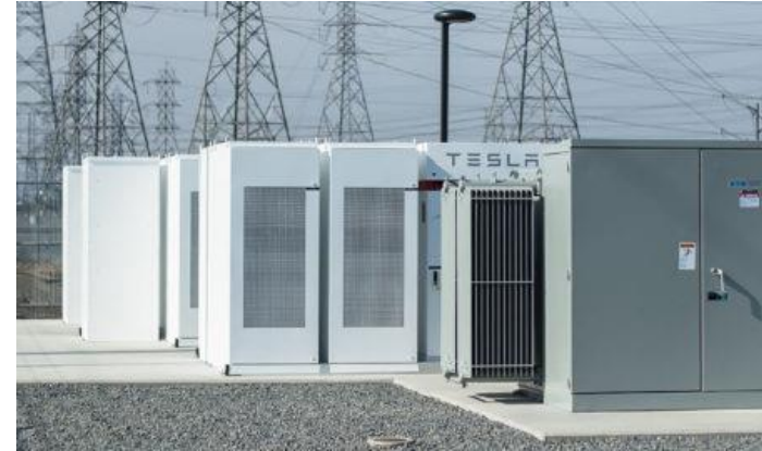
SCE/Tesla 20MW -80MWh Mira Loma Battery Facility
