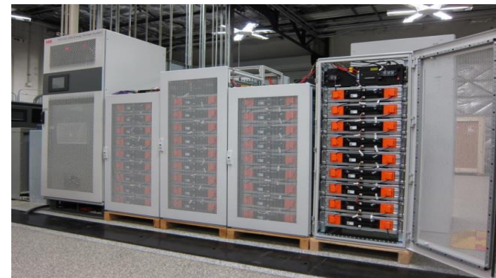
SCE Tehachapi plant, 8MW - 32MWh.
