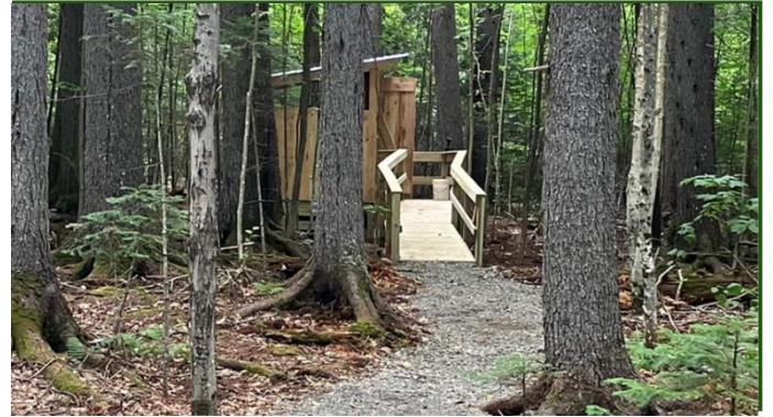
ADA-style moldering privy at Gravel Beach campsite on Chamberlain Lake, built by the NFCT crew and volunteers.
